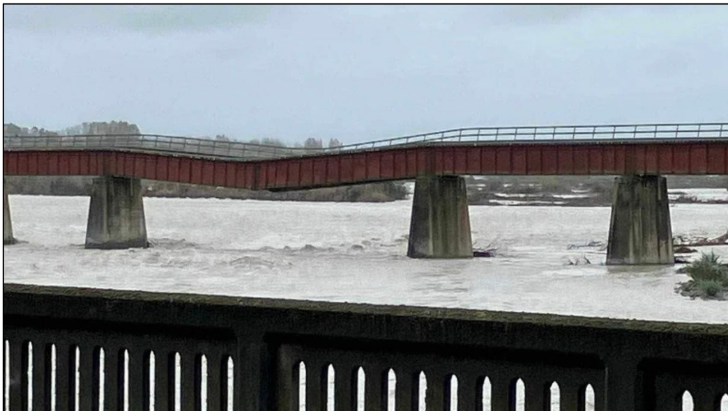
Figure 5: Collapsed Bridge 57 (12 April 2024)
