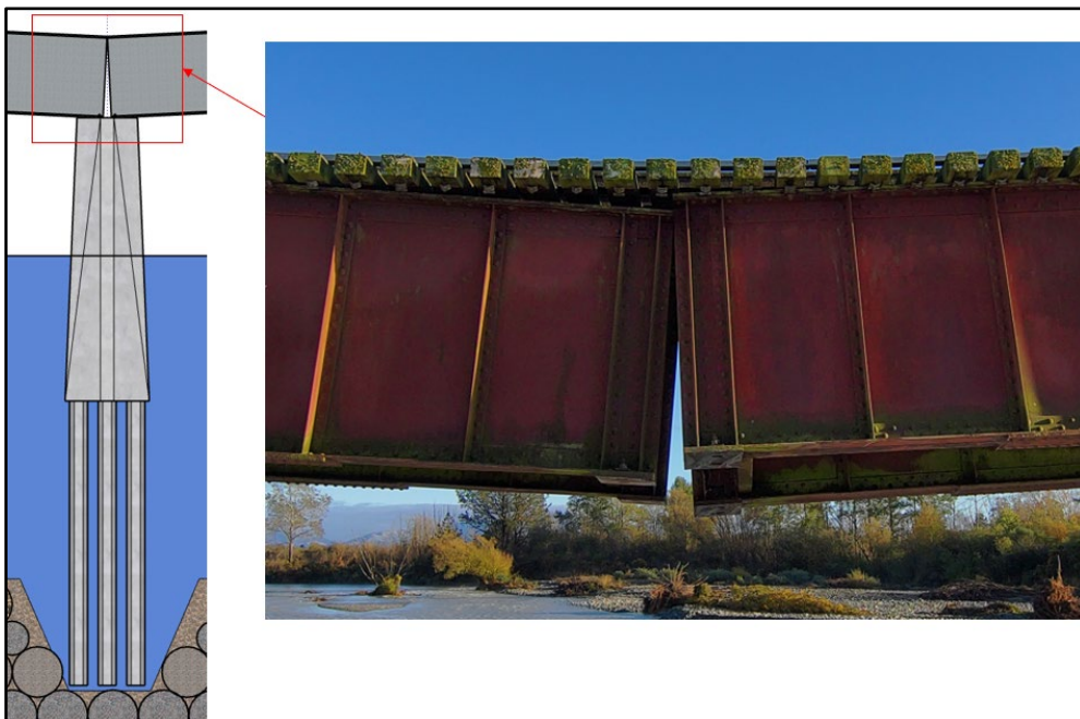
Figure 14: Vertical settlement of pier
