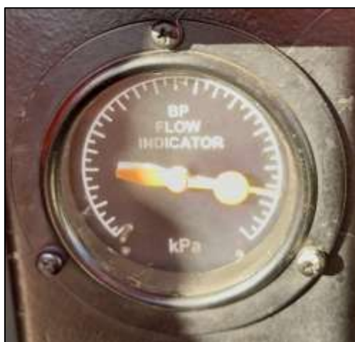
Figure 23: In-cab air-flow gauge at point of equalisation
