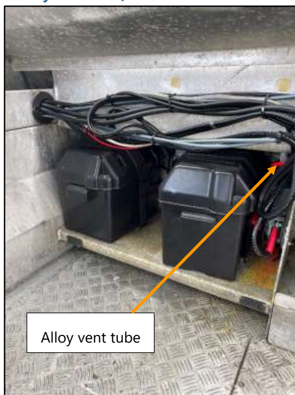
Figure 12: Location of alloy vent (after accident)
