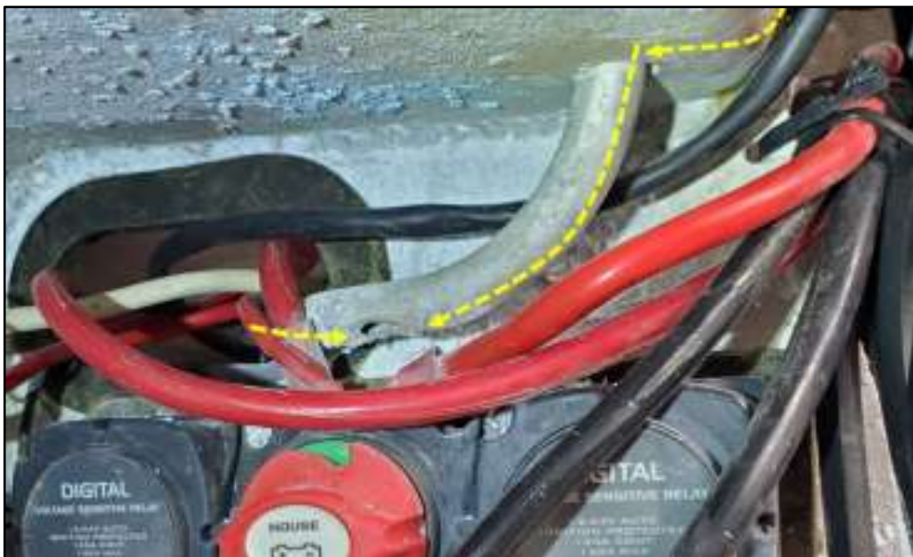
Figure 24: Low point of alloy vent tube (Credit: Quest Integrity)
