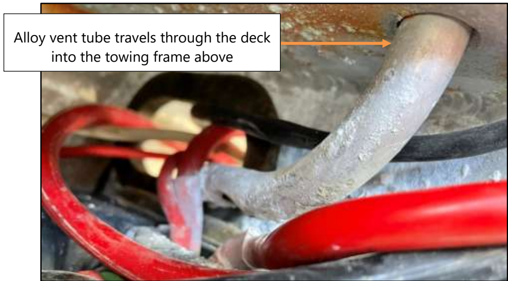
Figure 14: Alloy vent tube joining towing frame
