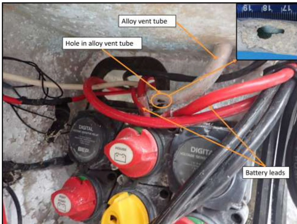
Figure 11: Hole in alloy vent tube (batteries removed for access after accident)
