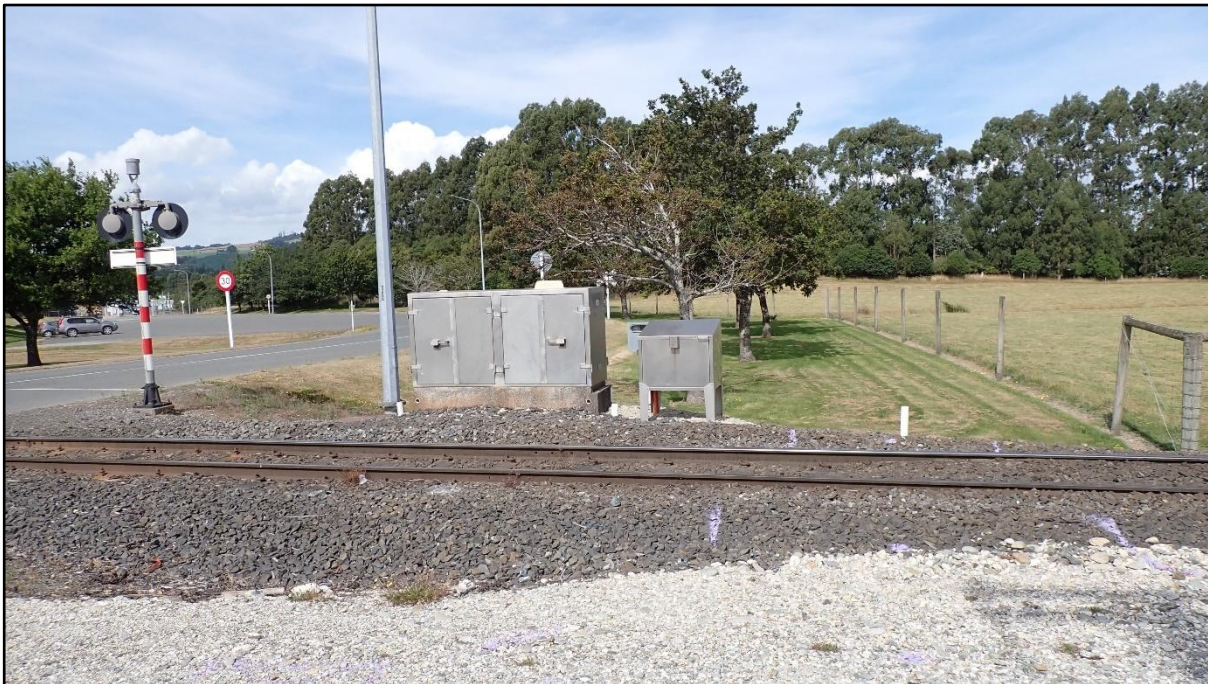
Figure 3: Signalling cabinet located near track at the crossing
