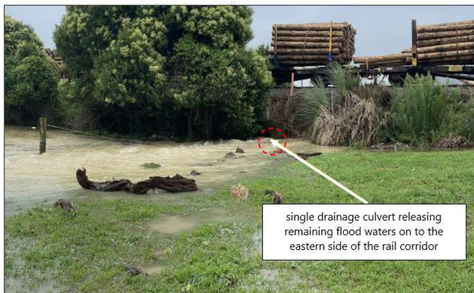
Figure 22: Culvert allowing floodwater to move east onto farmland (Credit: KiwiRail – photograph taken at approximately 10:00 on 29 January)
