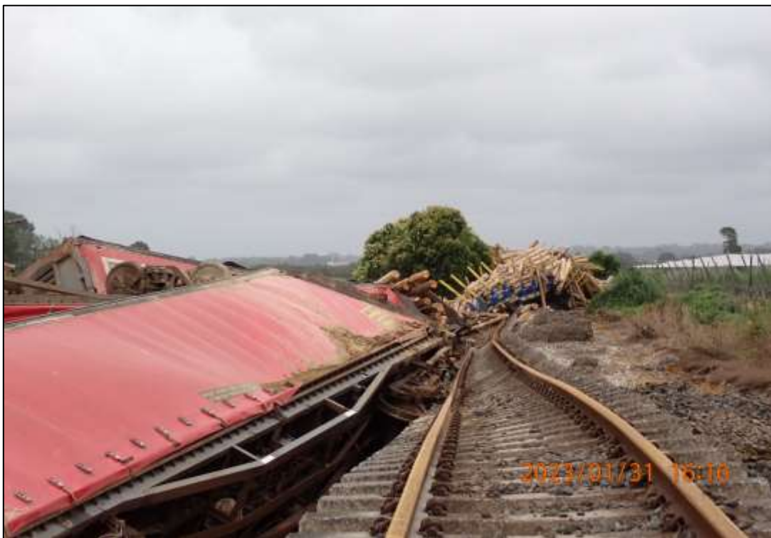
Figure 13: Derailed wagons and washed-out track formation
