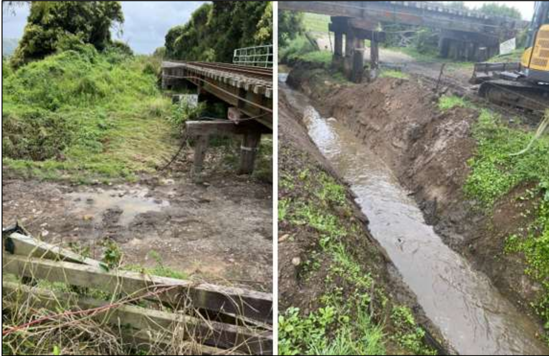
Figure 24: Remedial work at Bridge 85 after the accident (Credit: Bay of Plenty Regional Council)
