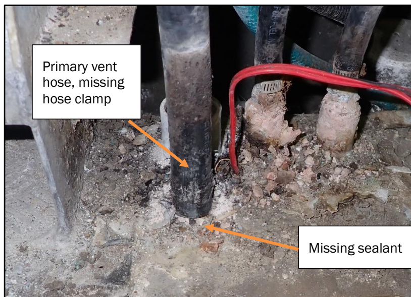
Figure 17: Primary vent hose connection to fuel tank (underneath the deck plate)
