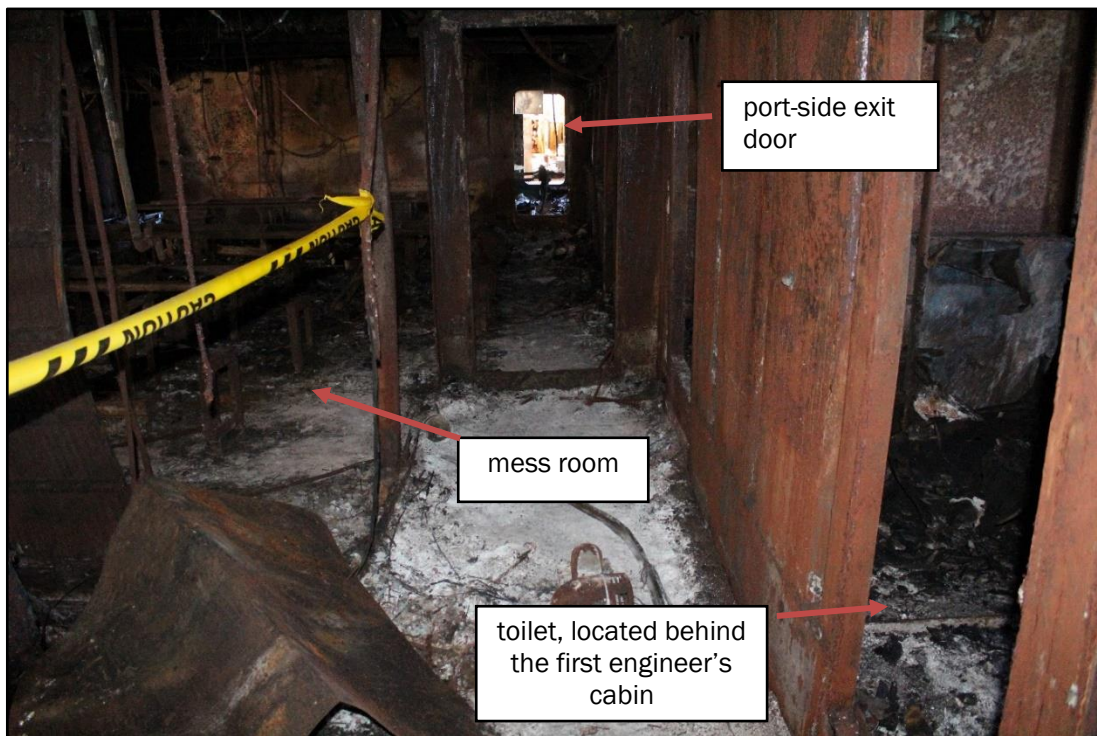
Figure 9: Fire damage to the officers' deck, port side
