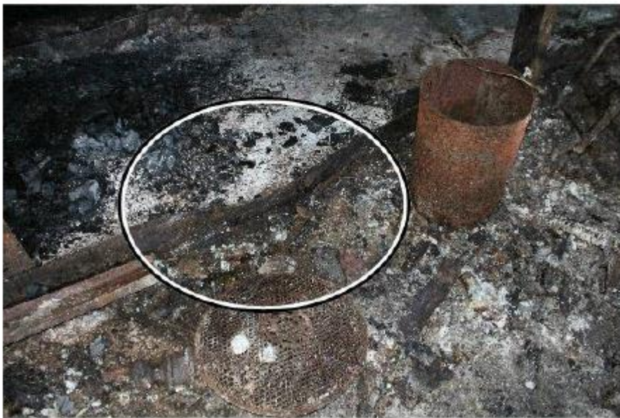
Photo 12: The circle shows the warped steel plate.
