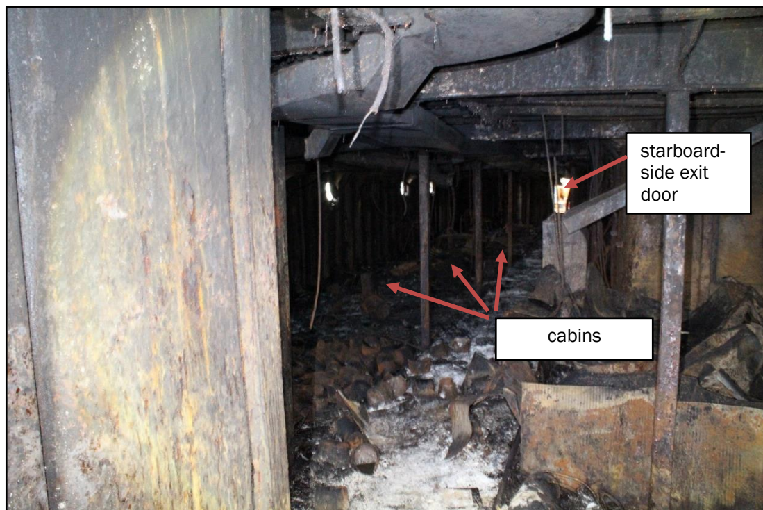
Figure 8: Fire damage to cabins on the officers' deck
