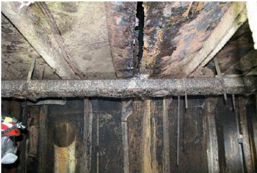
Photo 16: Shows the corrosion around the separation between the wall and ceiling in the Seamen's Living Quarters.
