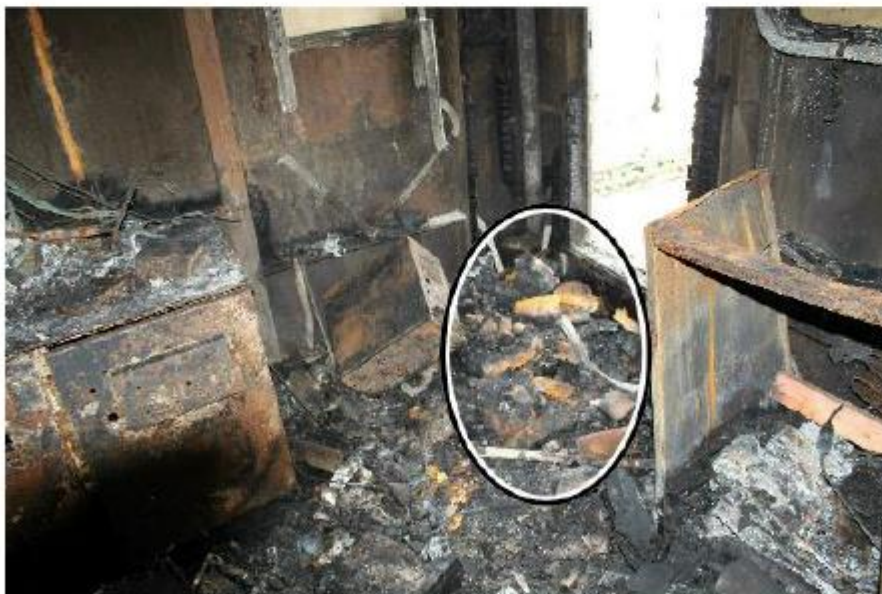
Photo 8: The circle shows the wall cladding and remaining floor at the rear entrance on the starboard side of the bridge.
