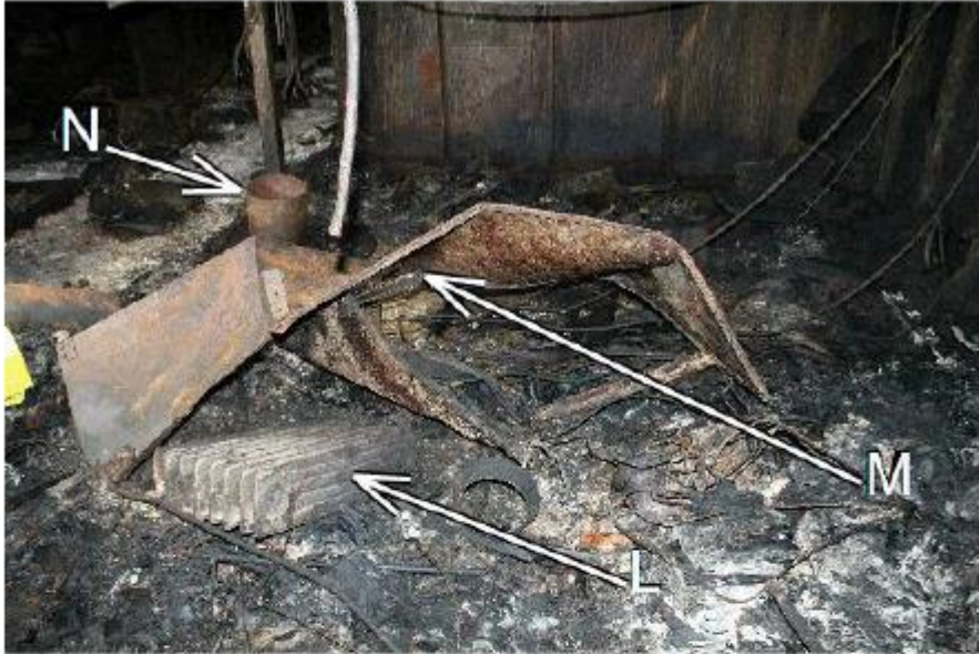
Photo 11: Shows the first engineer's cabin looking to the rear of it. 'M' identifies the fridge. Note the way it has collapsed. 'L' identifies the oil column heater. 'N' identifies the rubbish bin.
