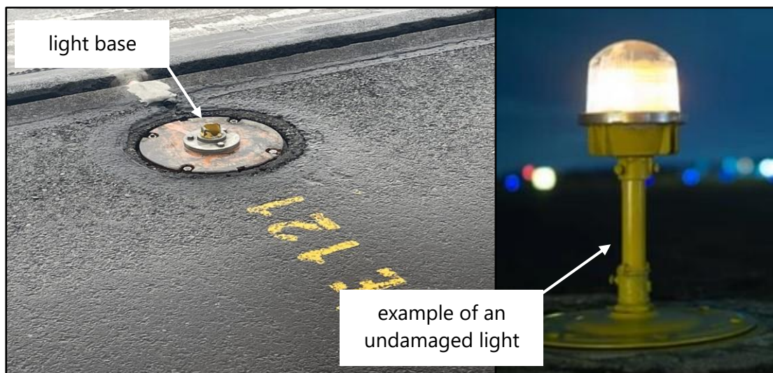
Figure 6: Runway edge lights
