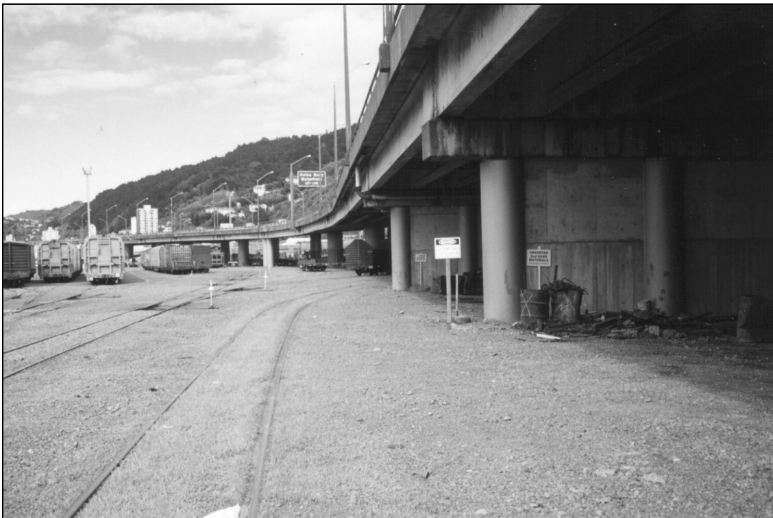
Figure 2 The view from the middle ferry shunt 40 m before the point of impact
