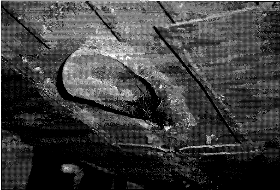
Figure 6 Damaged stern tube after removal of propeller shaft Note exposed remains of old heat exchanger
