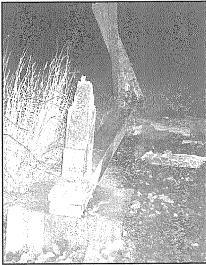
Bridge 355 (footbridge) pier following collision
