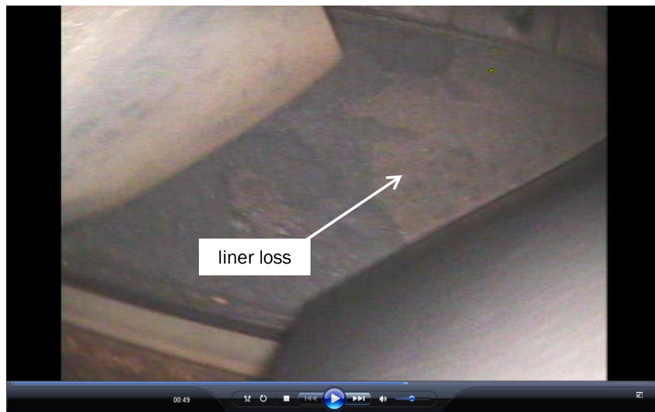
Figure 4 High-pressure compressor stage 1 compressor lining
