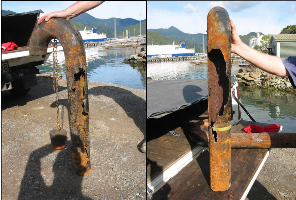
Figure 3 2 of the 3 wasted air pipes
