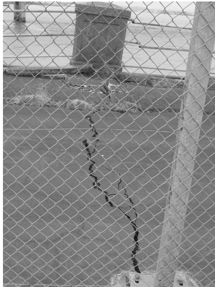
Figure 7 Damage to the old Mangere Bridge in the area of the second pier
