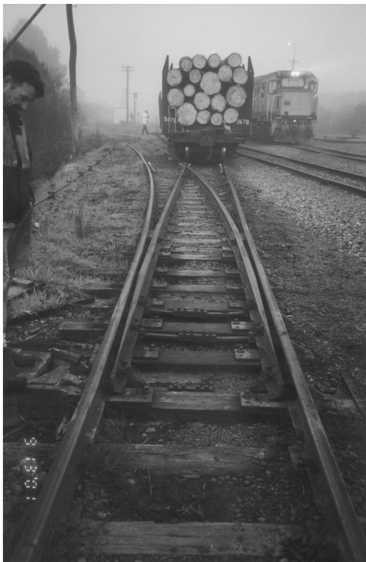
Figure 3 Looking west from the turnout which initiated the derailment, showing both switches open
